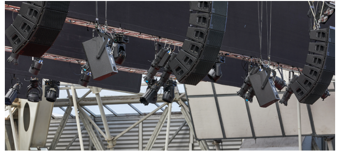
Y10P loudspeakers of the acoustic shell and Y8/Y12 main system on the front truss
